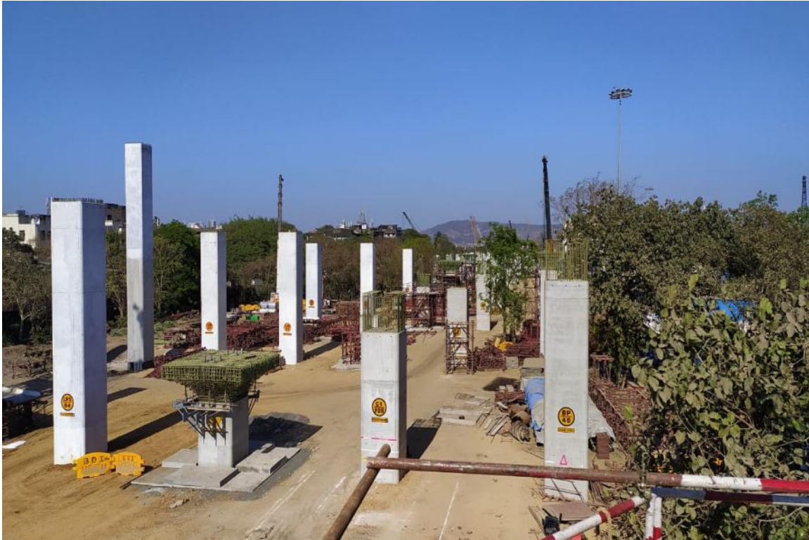
Photo No. 9: A View of Pier and Pier Caps at the Interchange Area
