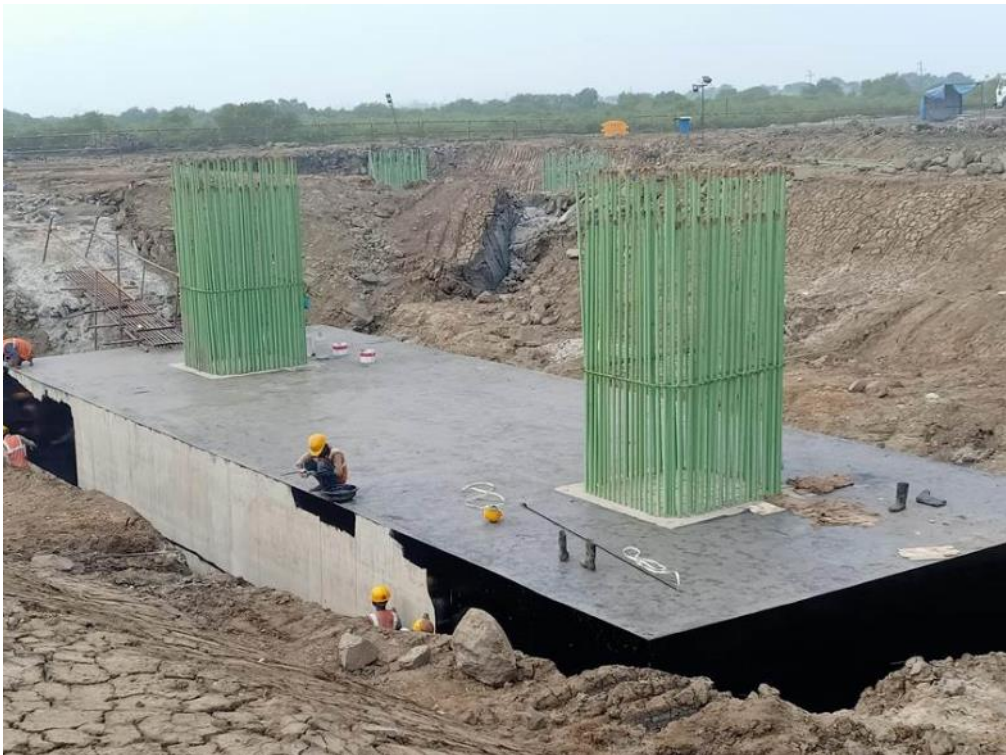
Photo No. 10: Coal Tar epoxy application at Open foundation MP 245 LHS in progress
