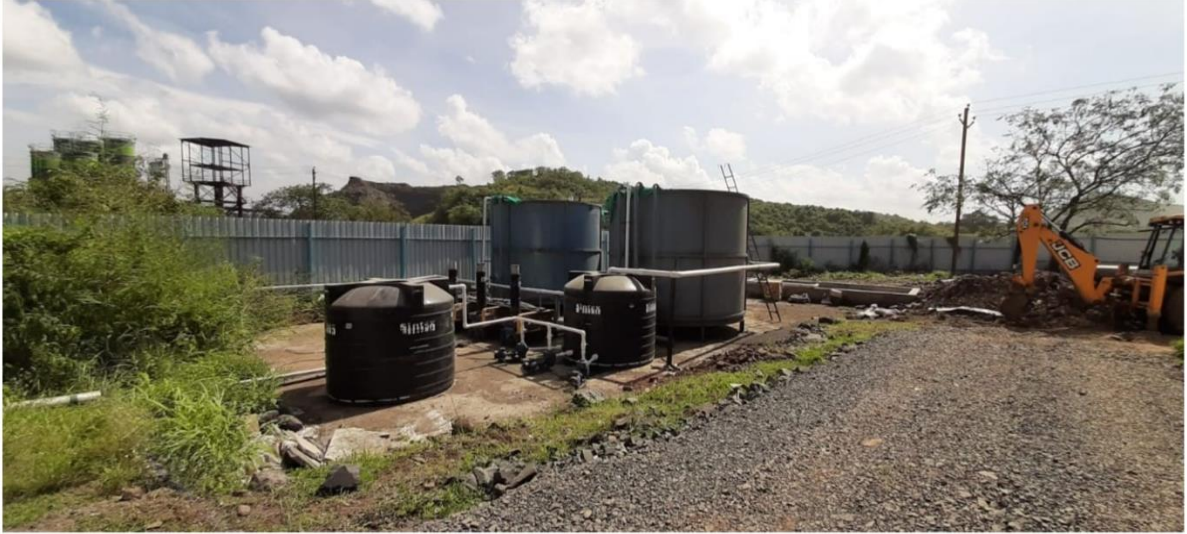
Sewage treatment plant at labour camp
