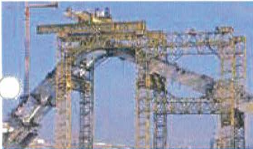
Sheik Zayed Bridge, Abu Dhabi - UAE (2009) Turning and lifting bridge segments to final position.
