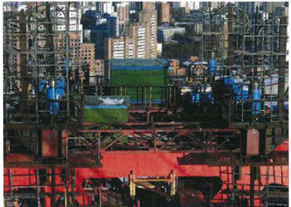
Serebryany Bor-Moskau-Ru Bridge - Russia (2008) VSL Heavy lifting units with hydraulic pumps and strands
