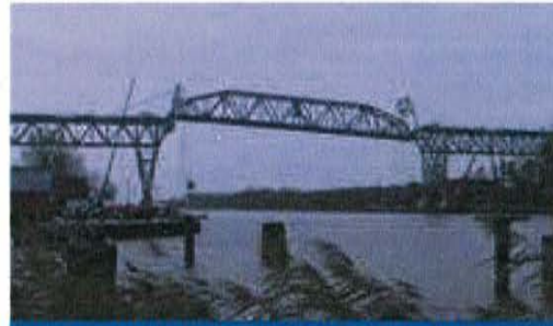
Hochdonn Railway Bridge - Germany (2006) Lowering of the steel structure (1.465t, lifting and tilting operations).
