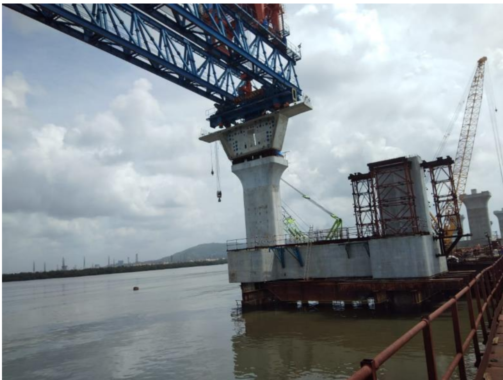
Photo No. 12: MP-19 N Pier Head Segment Erection - Intertidal Section in progress
