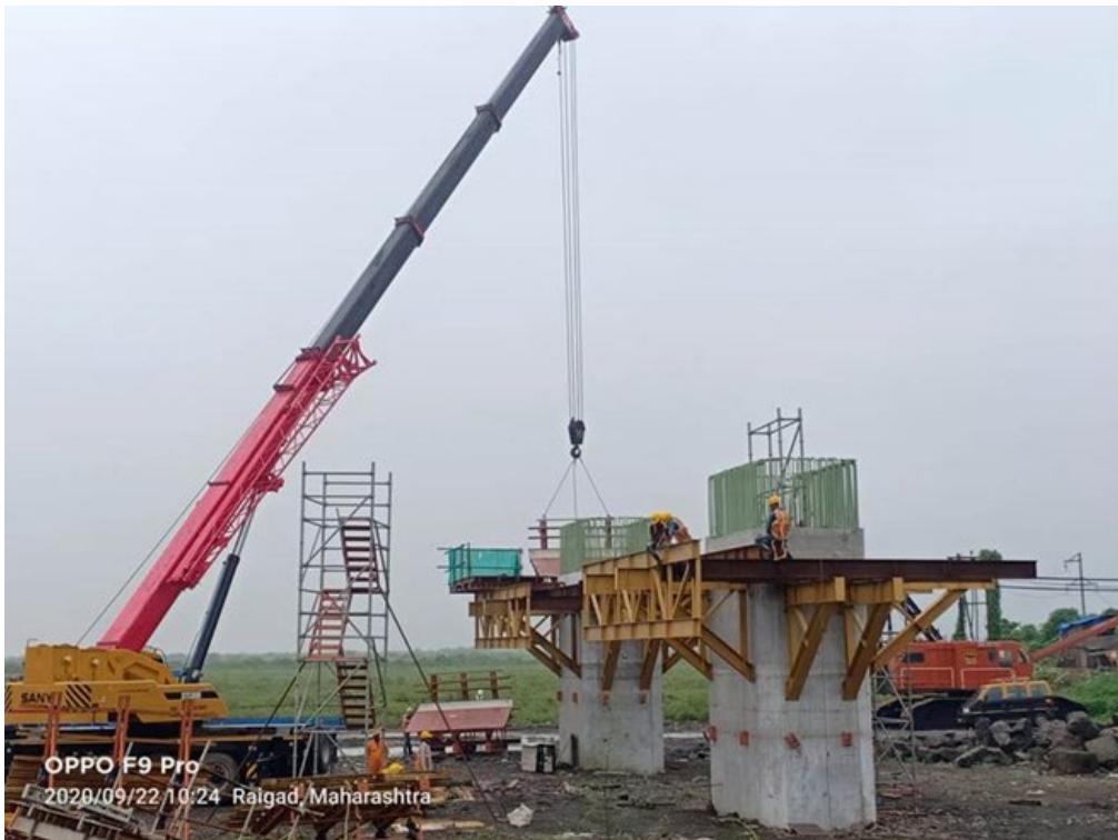
Photo No. 4: Pier Cap bottom formwork preparatory works at MP 241 LHS and RHS in progress
