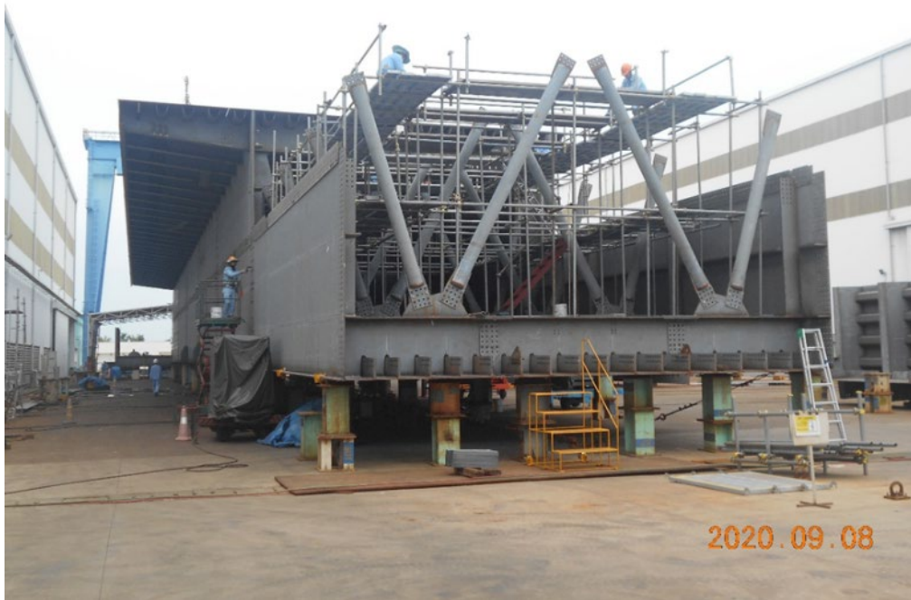
Photo No. 6: Trial Assembly of OSD Girder Bridge P1-OS04-NG (Lot6) / Seg. 28~32 in Vietnam in progress
