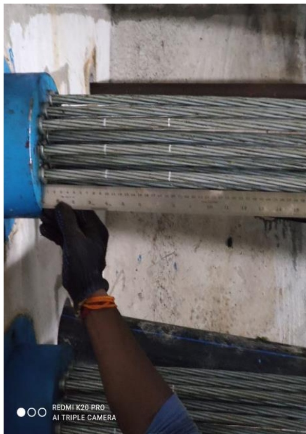
Photo No. 8: Slip Check After 24 Hrs of Stressing at MP17-18 N Tendons in progress
