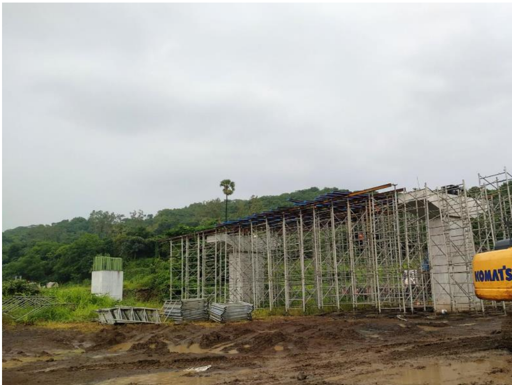
Photo No. 12: Staging Arrangement for Cast in-situ voided slab of span MJP-7 to 8 (Chirle) in progress
