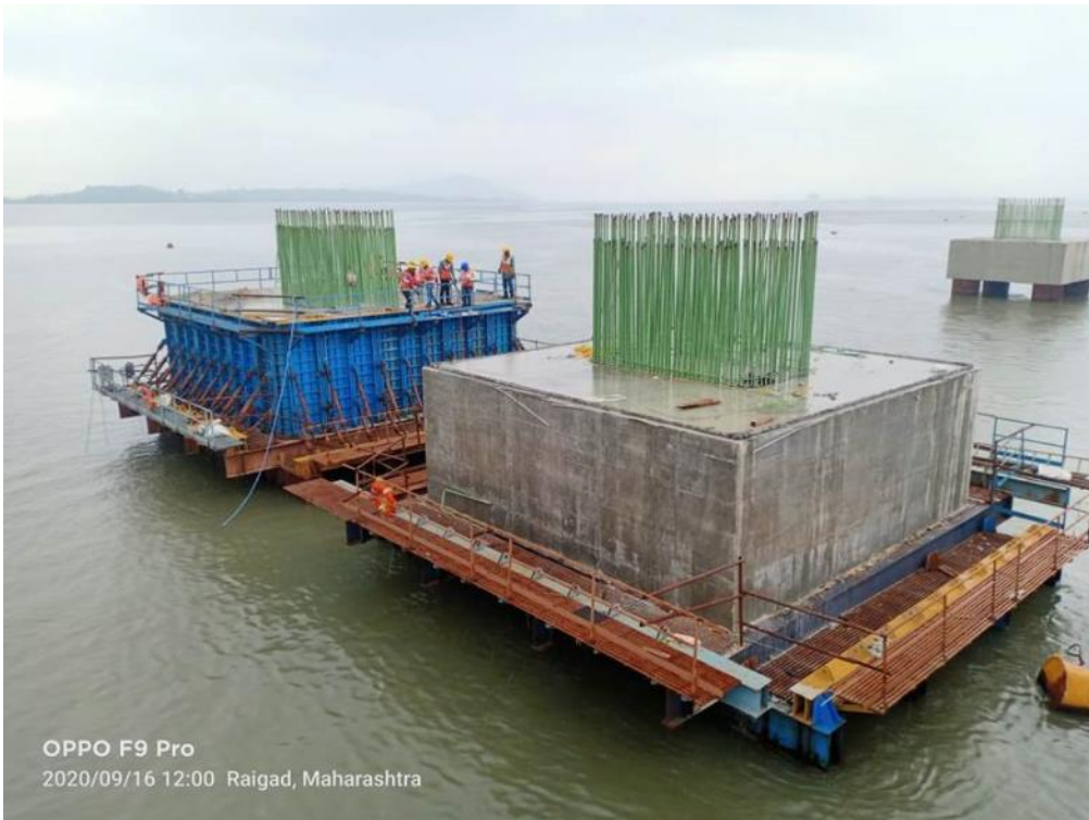
Photo No. 10: Pile Cap curing Works at MP 212 LHS and RHS in progress
