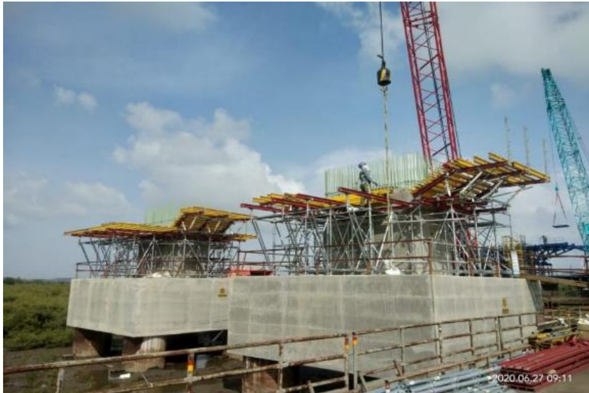
Photo No. 3: Pier cap formwork at MP238 LHS and RHS in progress
