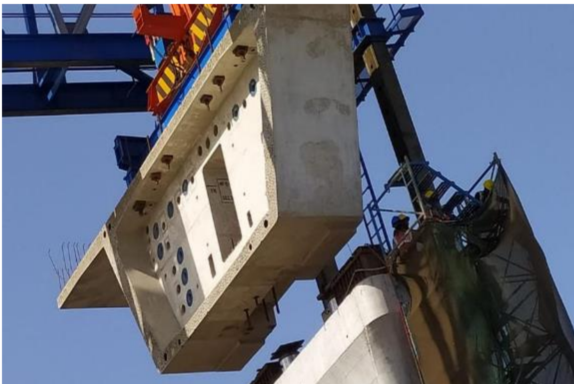
Photo No. 4: MP15-16 N Pier Head Erection at Intertidal Section in progress
