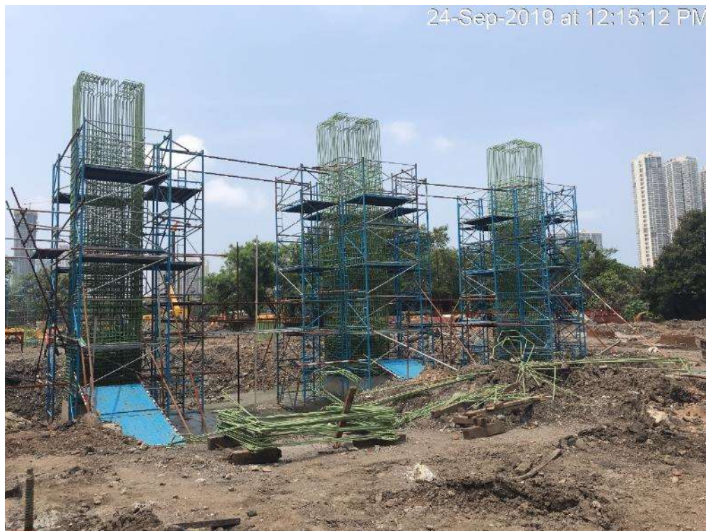
Photo No. 6: Reinforcement work for Pier at the interchange location is in progress
