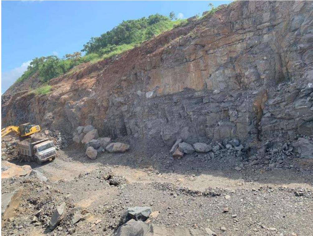
Photo No. 9: Excavated material shifting at At-grade area Ch @ 19+720 is in progress
