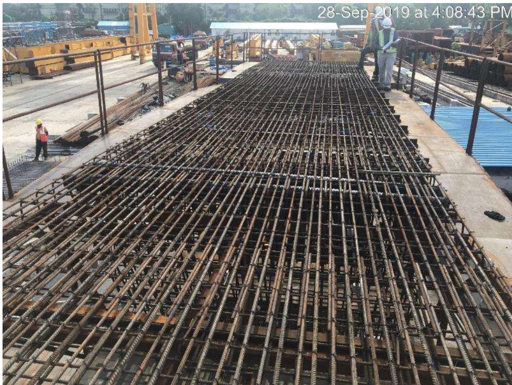
Photo No. 8: Reinforcement Inspection at Zig of Segment 88-89 NS4 is in progress
