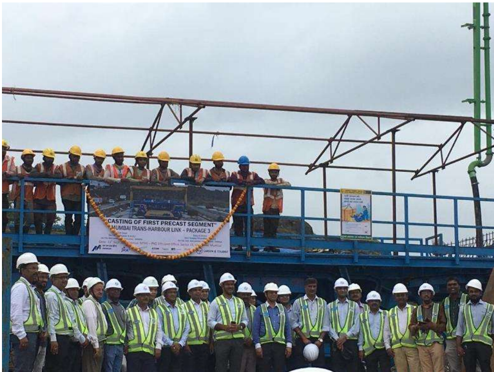
Photo No. 10: First precast Segment Casting Ceremony at the Pkg-3 Precast yard dated 11 th Sept. 2019
