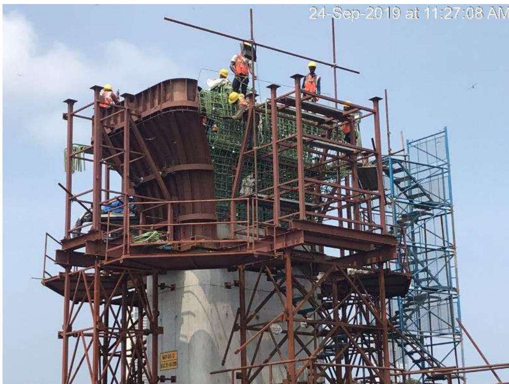
Photo No. 2: Pier cap shuttering work at MP-06 N is in progress
