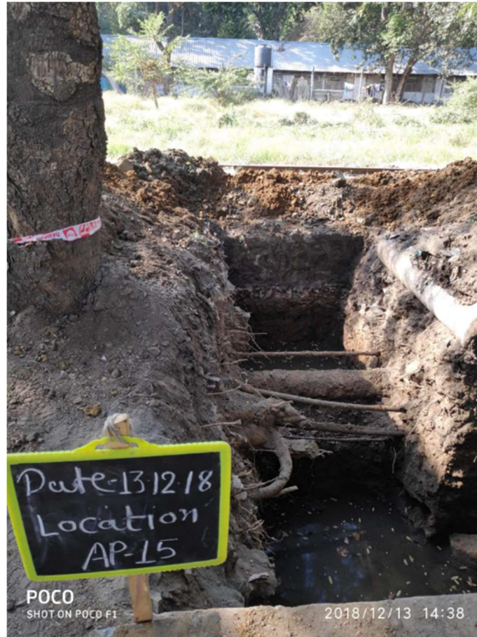
Photo No. 13: Trenching Works for physically identifying the utilities at AP 15 Location
