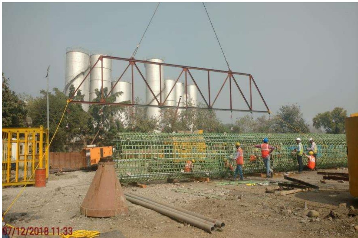
Photo No. 6: Reinforcement cage erection for Test Piling in intertidal portion in progress
