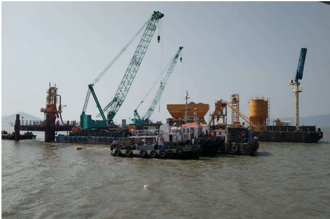
Photo No. 20: Overall set-up view of Test Pile at Location MP 179 L
