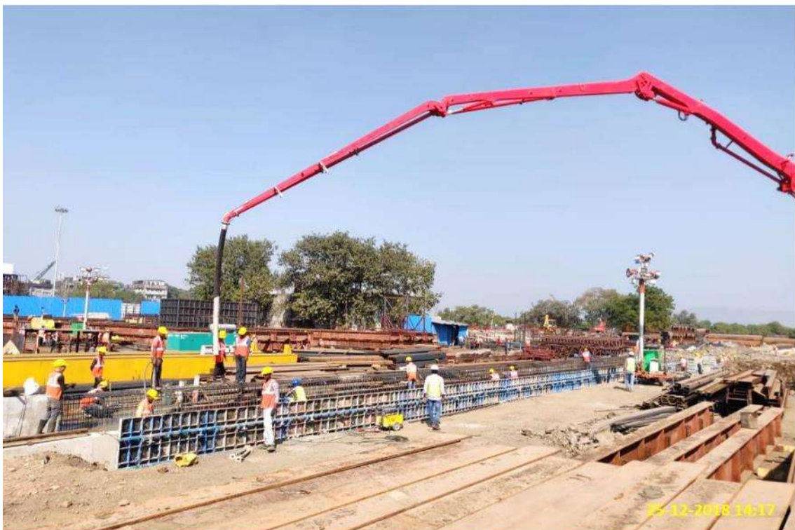
Photo No. 14: Gantry Track Foundation Casting Works at STP Yard in progress
