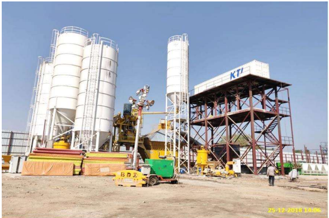
Photo No. 10: M1T Batching Plant commissioned at STP Yard
