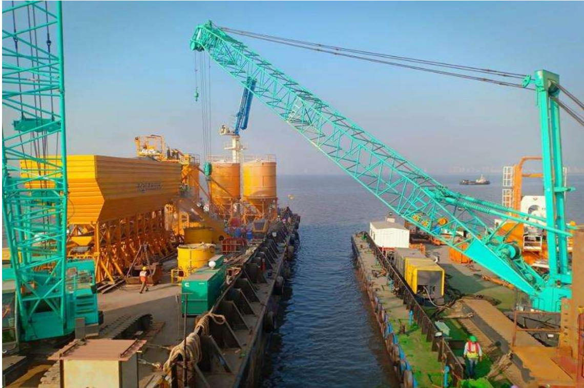
Photo No. 19: Marine Batching Plant Set-up
