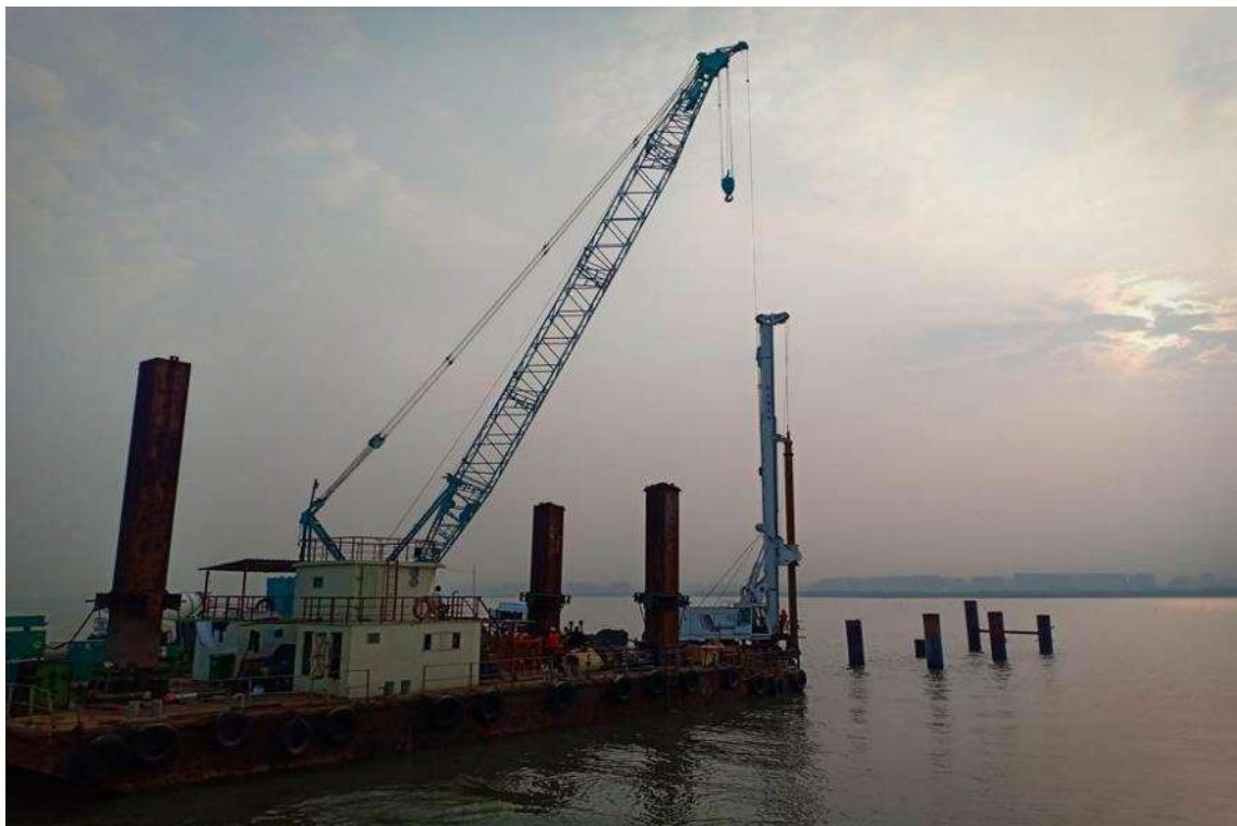
Photo No. 16: Temporary Access Bridge (TAB) – Front Side Piling works in progress
