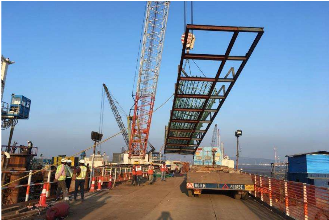
Photo No. 5: Reinforcement cage erection for Test Piling in intertidal portion in progress
