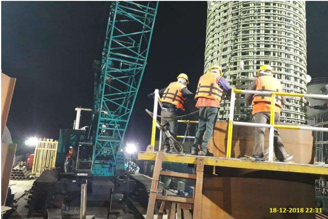
Photo No. 7: Reinforcement cage installation at MP 95 in Marine Portion in progress
