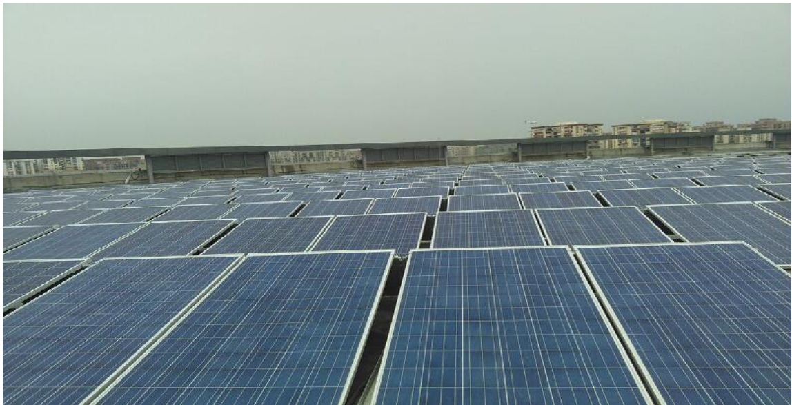
Solar PV Power panel
