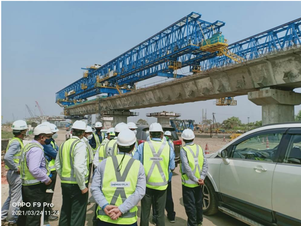
Photo No. 1: The DB Members & MMRDA officials visited the Pkg-2 site on 24 th March 2021
