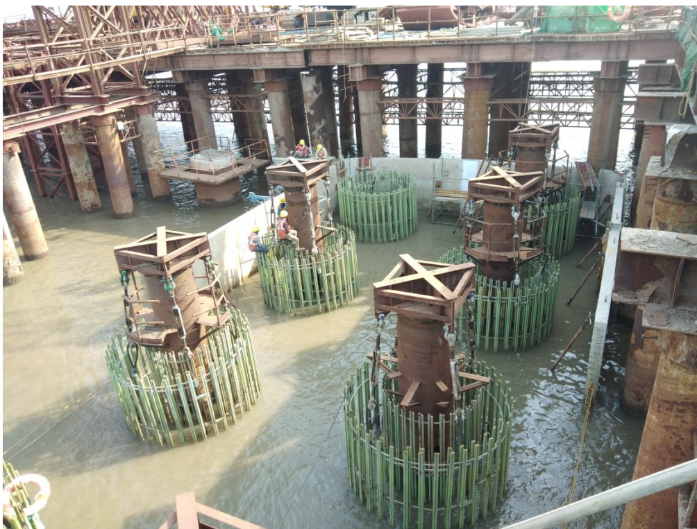
Photo No. 2: MP 52 OSD Pile Cap Works at the Marine Section in progress
