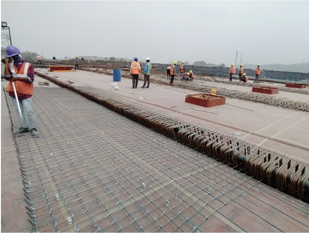
Photo No. 9: RP4-3 Cast in-situ 3 cell box girder Deck slab reinforcement in progress
