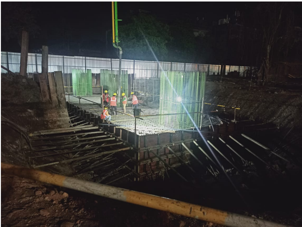
Photo No. 4: Casting of combined Pile cap at Interchange Section in progress
