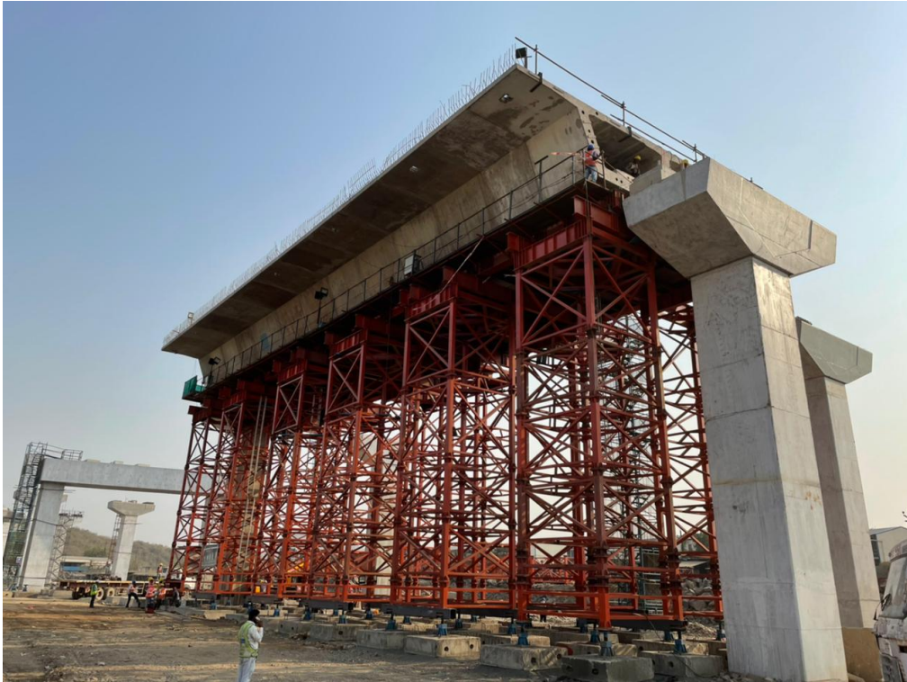
Photo No. 11: Span LMP 277-278, Segment gluing and temporary pre-stressing work in progress
