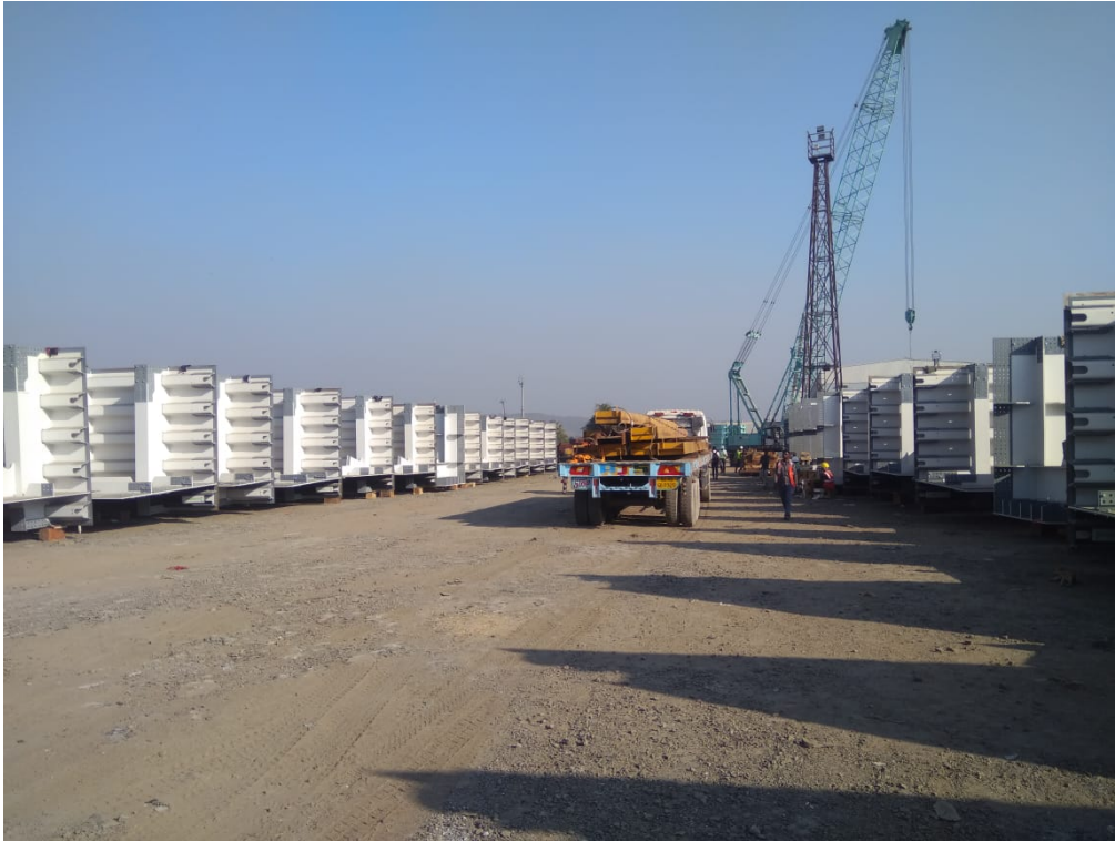
Photo No.7: Inward Material received for OSD 4- NG Fabricated Blocks 1st Lot., Segment No. 01 to 17, 203.2 m at Chirle Yard Site
