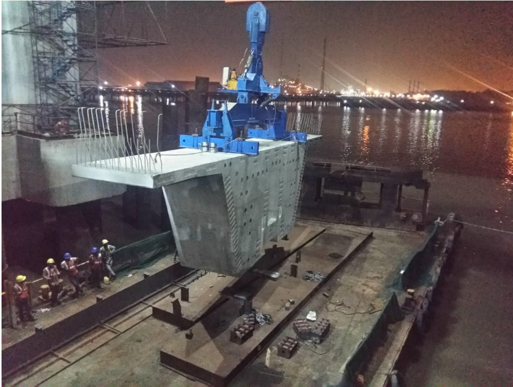
Photo No. 9: Erection of Pier segment for LG-03 at MP81 in progress
