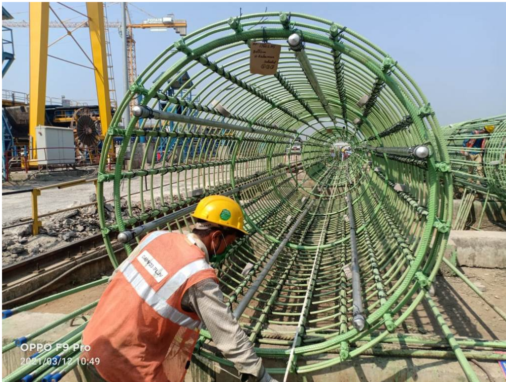
Photo No. 10: Pile reinforcement cage inspection at the Casting Yard in progress
