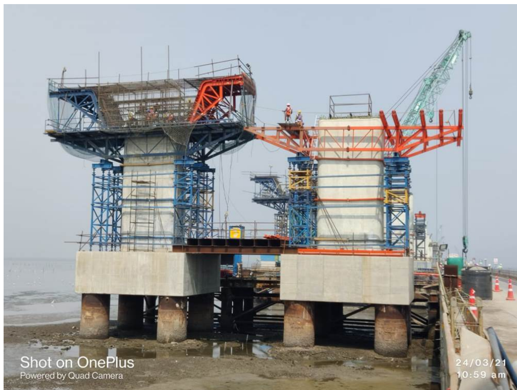
Photo No. 2: Pier head segment scaffolding and reinforcement at MP 229 LHS and RHS respectively in progress
