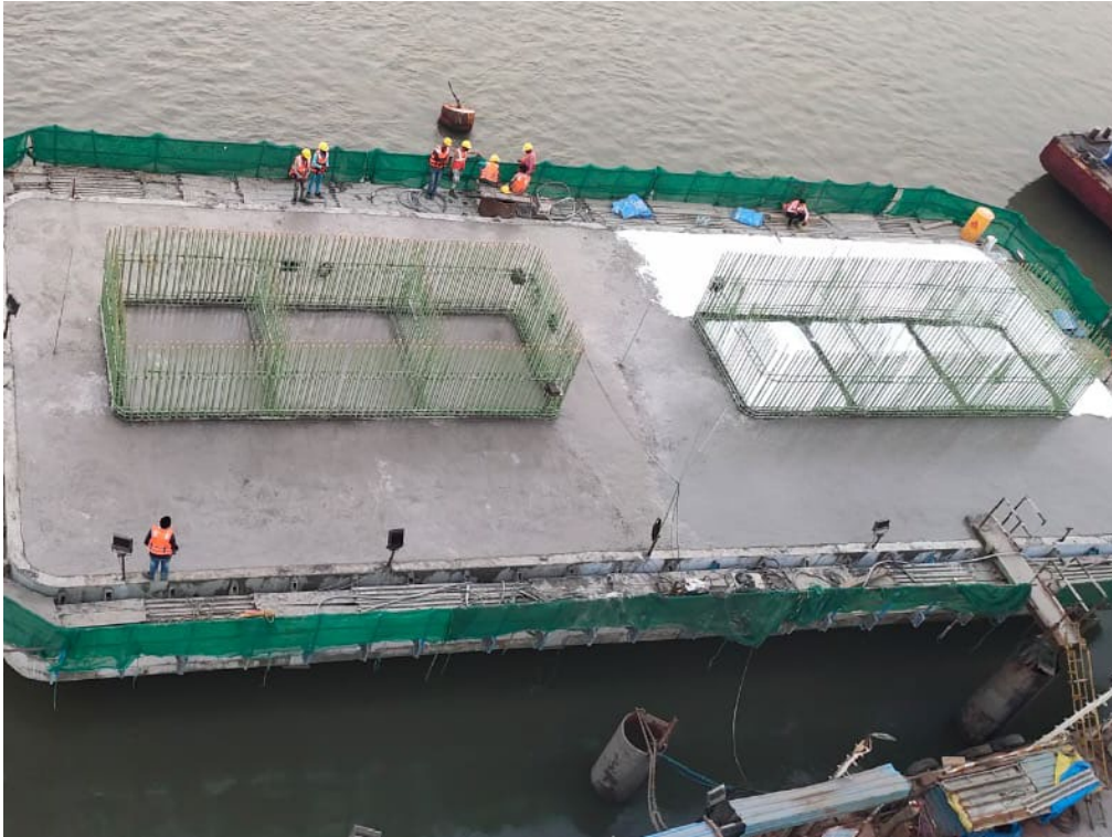
Photo No. 3: Casting of OSD Pile Cap at MP125 – Marine Section in progress
