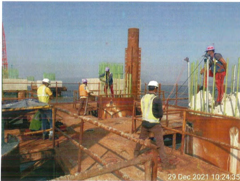
Photo No. 4: Sonic Tube Testing in progress at MP 170 RHS in progress
