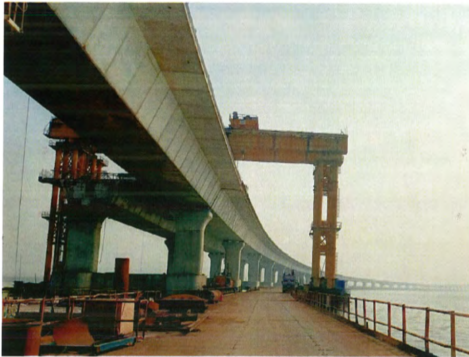
Photo No. 3: A view of the erected spans at the intertidal area (MP 11 to MP 50) looking towards Navi Mumbai
