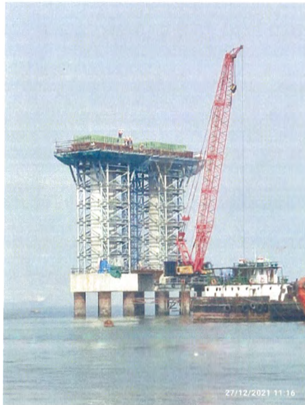
Photo No. 6: OSD Pier Cap reinforcement tying at MP 180 LHS and RHS in progress
