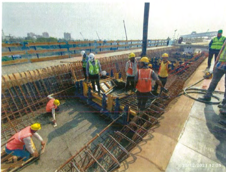
Photo No. 8: Cast in situ bottom slab concreting at Ramp MA in progress
