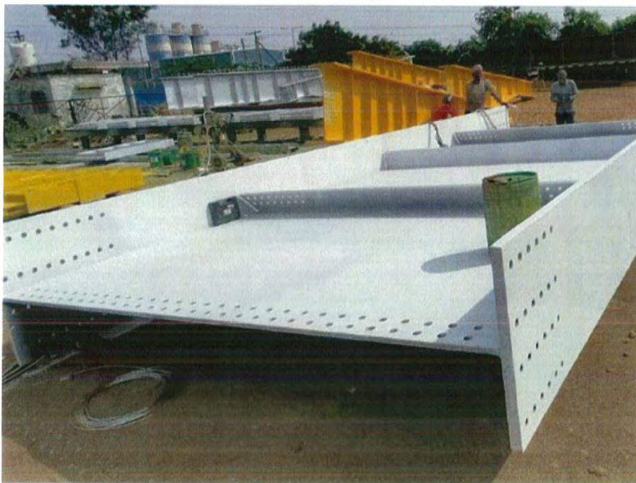
Photo No. 10: ROB Girder Structure Steel Painting at Global Steel Company in progress
