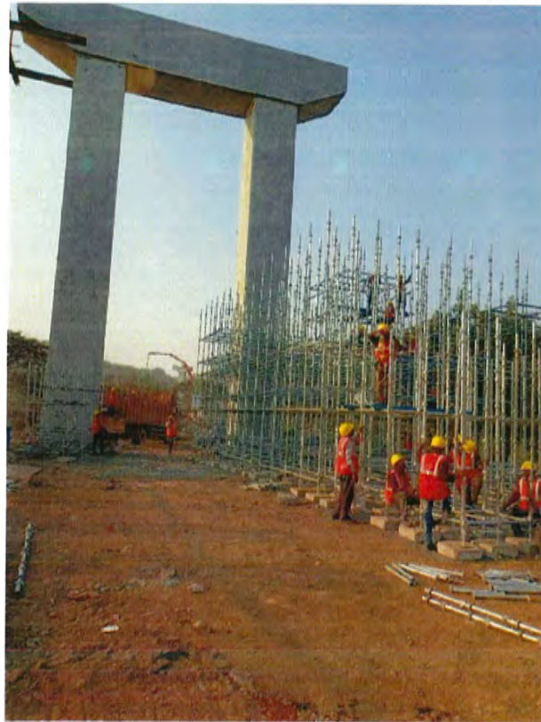
Photo No. 11: Span LP 22-23 Staging work for Cast-in-situ 3 Cell box girder in progress
