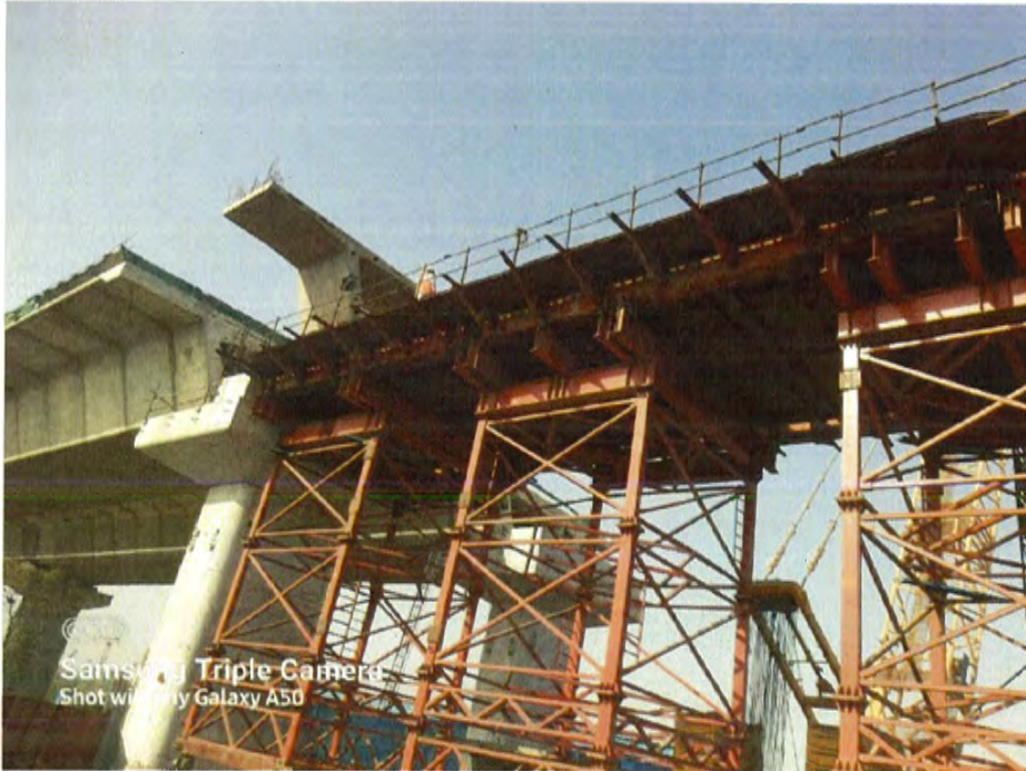
Photo No. 1: Gavan Span RMP 266-267, interface location, segment erection work in progress
