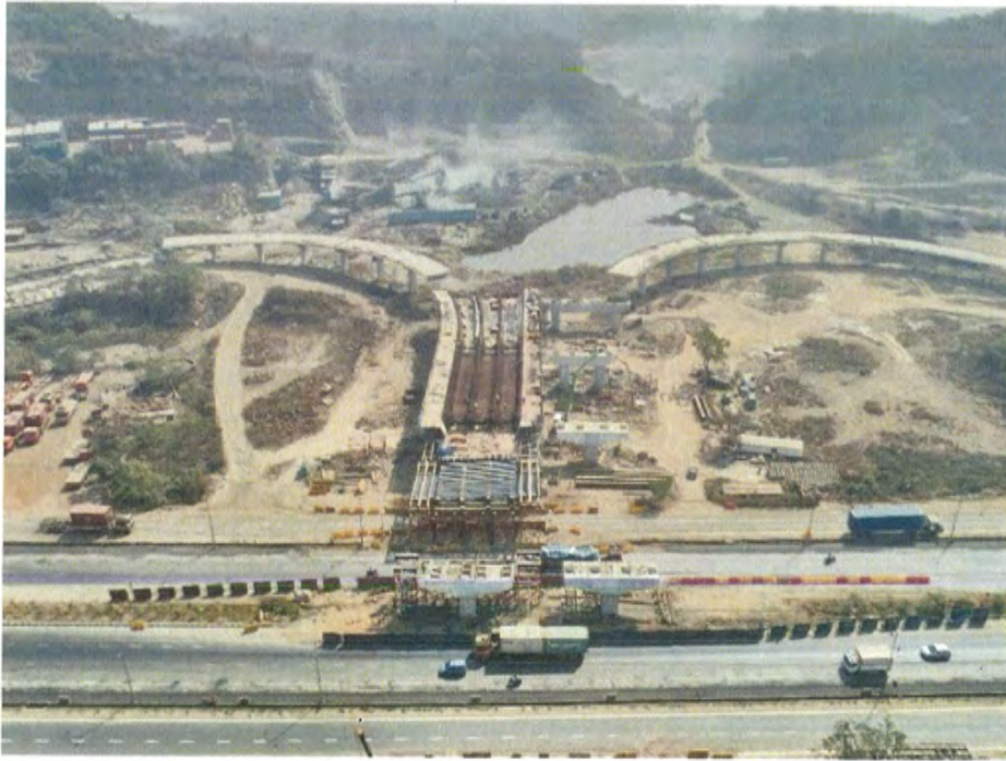
Photo No. 7: A view of MTHL Bridge – MJP & PMP Ramps at Chirle Interchange
