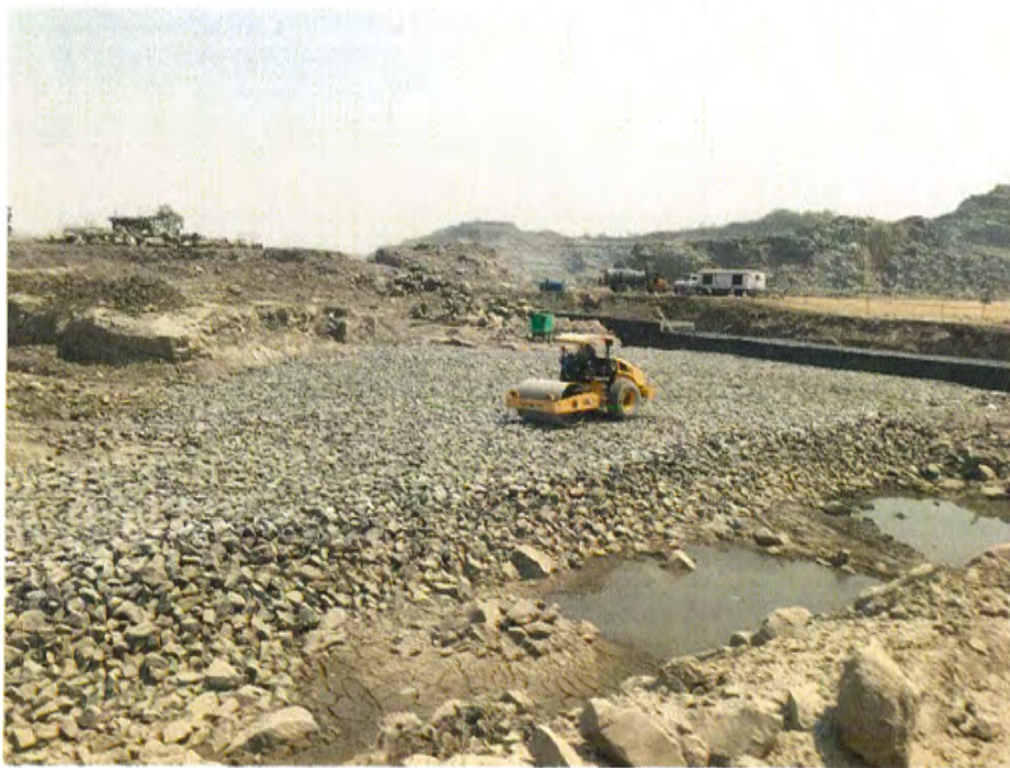
Photo No. 12: Rock fill embankment work at CH 19+440 to CH 19+500 RHS in progress
