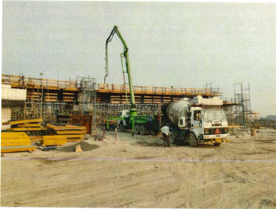
Photo No. 11: Cast in situ bottom slab concrete at Ramp AC Span ACP-7 to ACP-8 in progress
