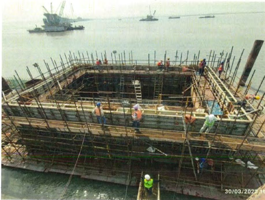
Photo No. 9: PC shell wall formwork alignment at MP 183 RHS in progress
