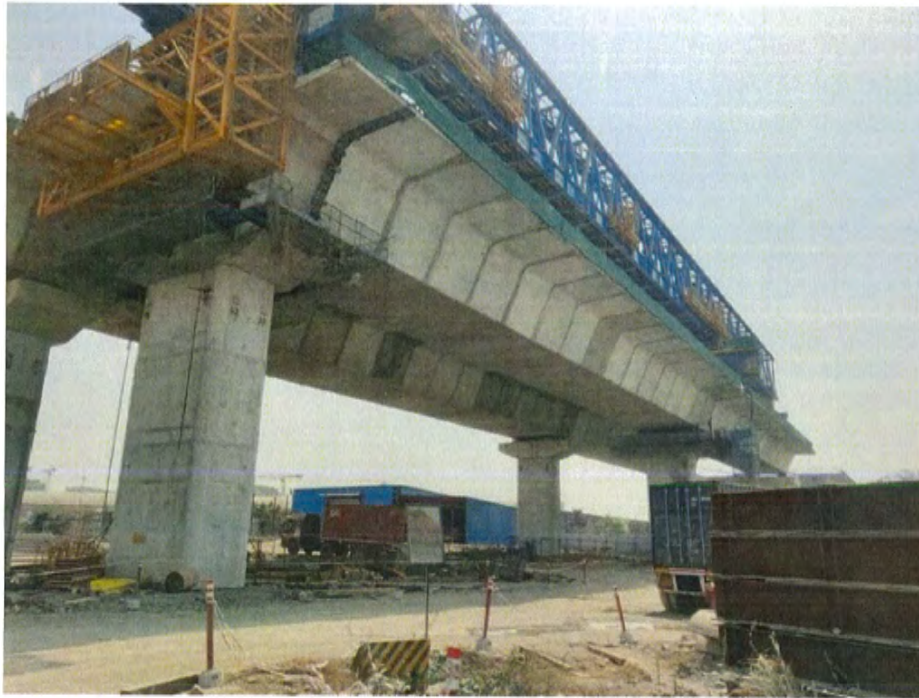
Photo No. 1: LG-3 Wet joint formwork fixing at Span MP 264-265 RHS in progress
