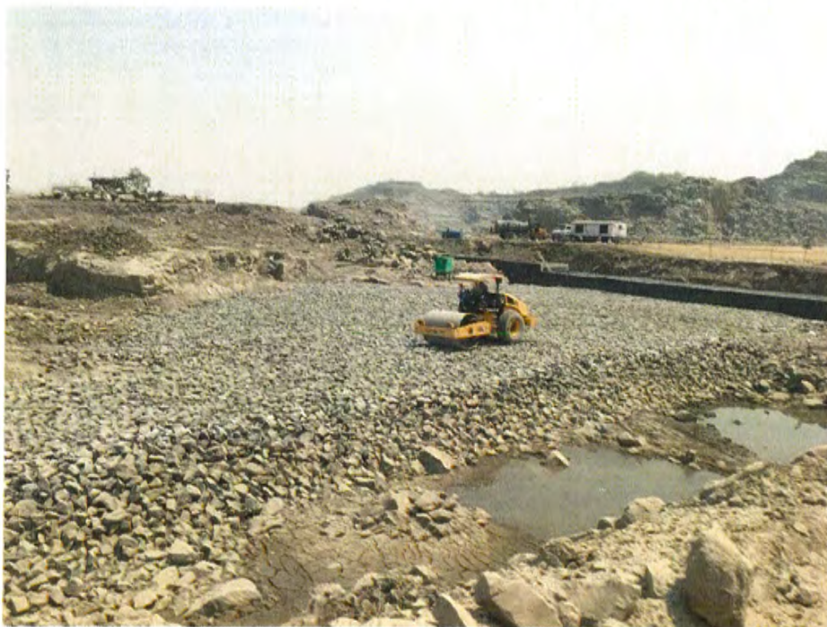
Photo No. 12: Rock fill embankment work at CH 19+440 to CH 19+500 RHS in progress
