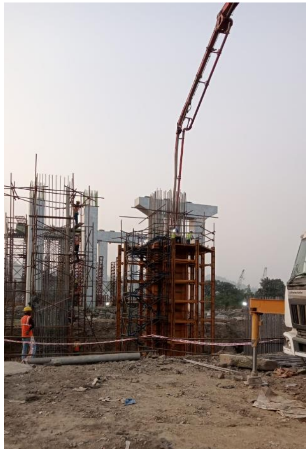
Photo No. 8: RP 24C pier 1st lift 6.5m concrete pouring work in progress
