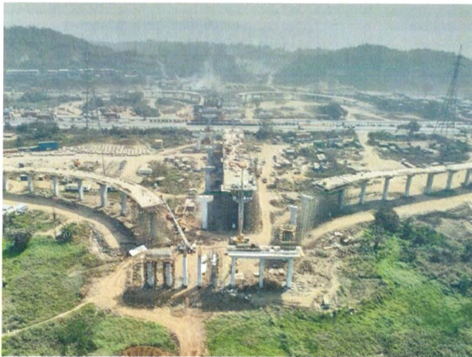
Photo No. 6: A view of MTHL Bridge – MPP & JMP Ramps at Chirle Interchange
