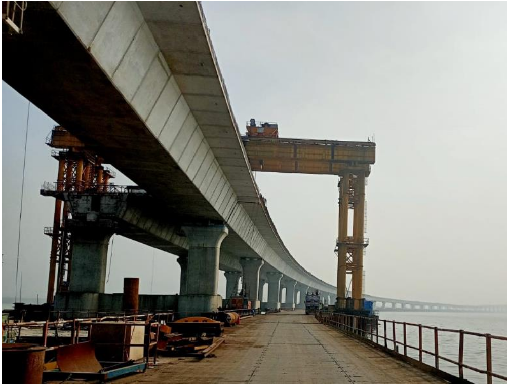
Photo No. 3: A view of the erected spans at the intertidal area (MP 11 to MP 50) looking towards Navi Mumbai
