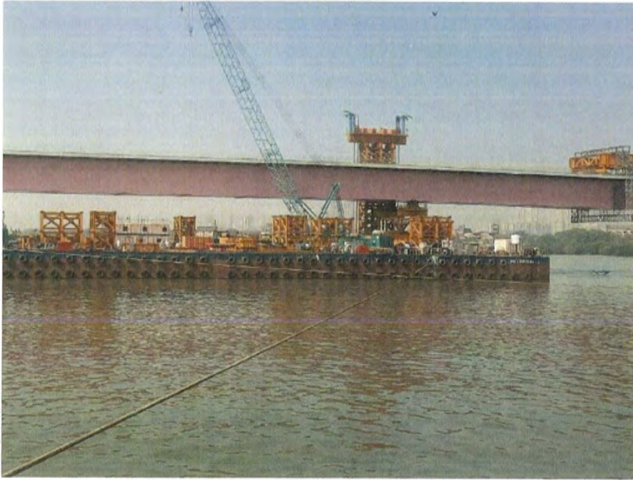
Photo No. 1: OSD 4 N span 3 Girder Transporting to MP 126 N through Barge
