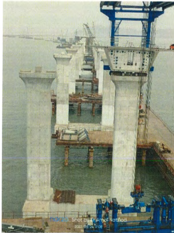
Photo No. 5: A view of MTHL Bridge taken from the LG-8 looking towards Navi Mumbai
