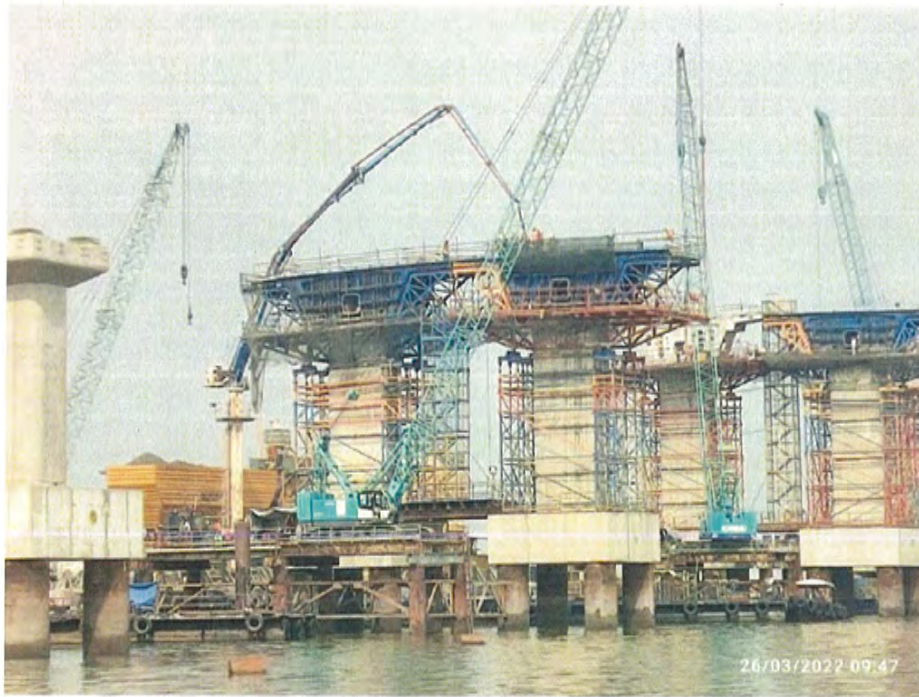
Photo No. 5: Integral Pier head segment concrete at MP 195 LHS in progress
