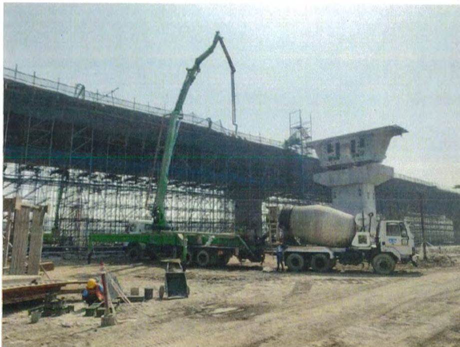
Photo No. 2: Cantilever slab and strut concrete in progress at Span MP 256-257 LHS
