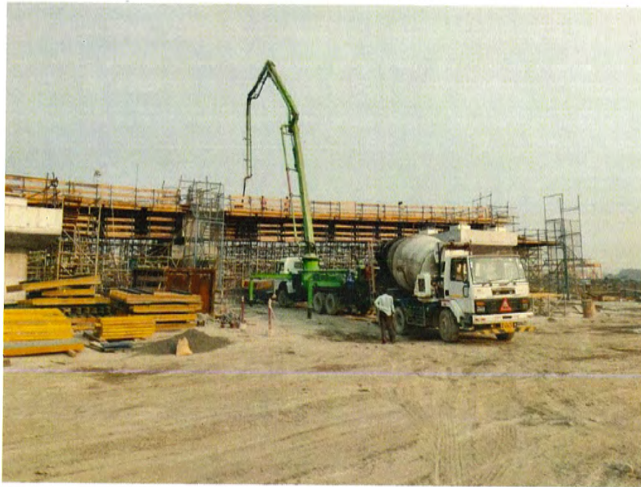
Photo No. 11: Cast in situ bottom slab concrete at Ramp AC Span ACP-7 to ACP-8 in progress
