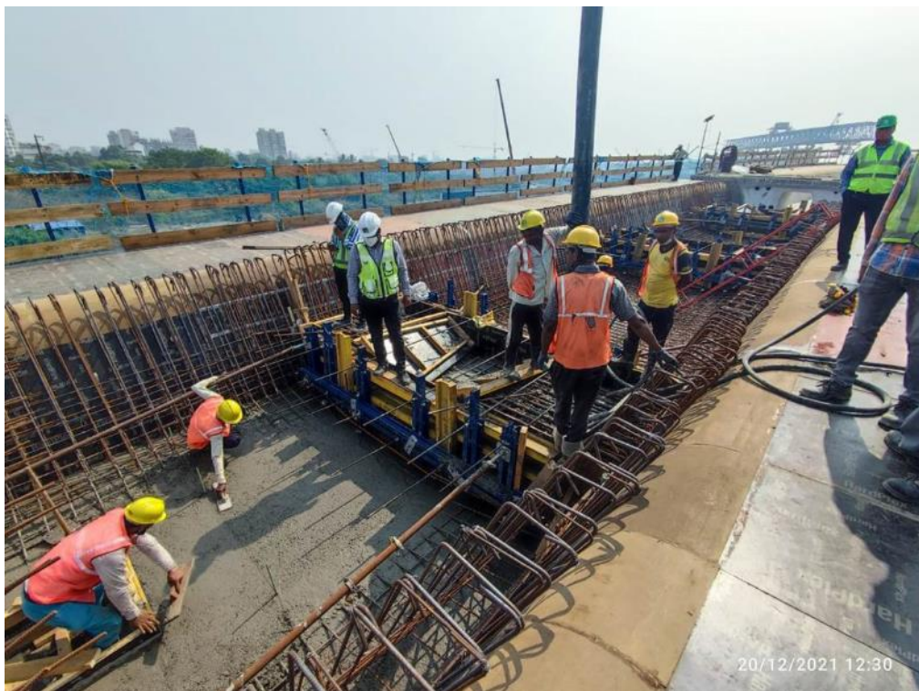
Photo No. 8: Cast in situ bottom slab concreting at Ramp MA in progress
