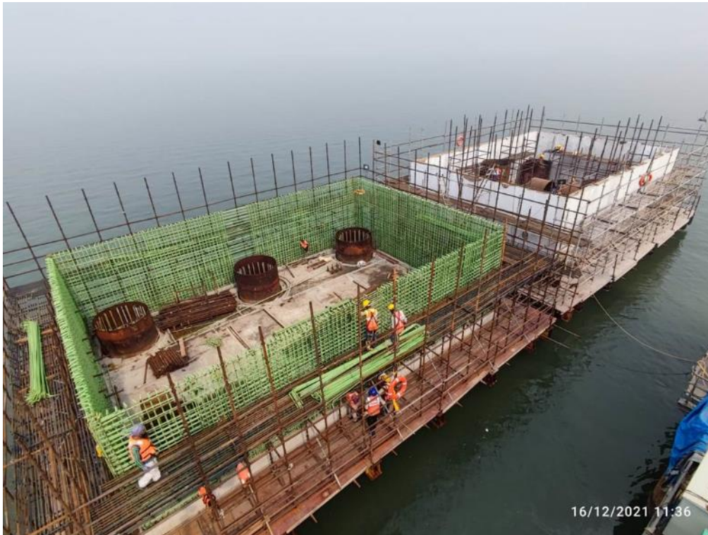
Photo No. 11: PC Shell wall reinforcement tying at MP 185 RHS in progress
