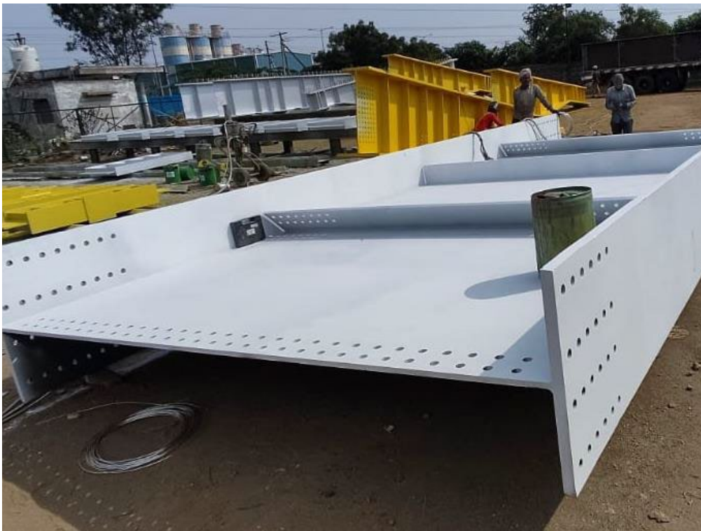
Photo No. 10: ROB Girder Structure Steel Painting at Global Steel Company in progress
