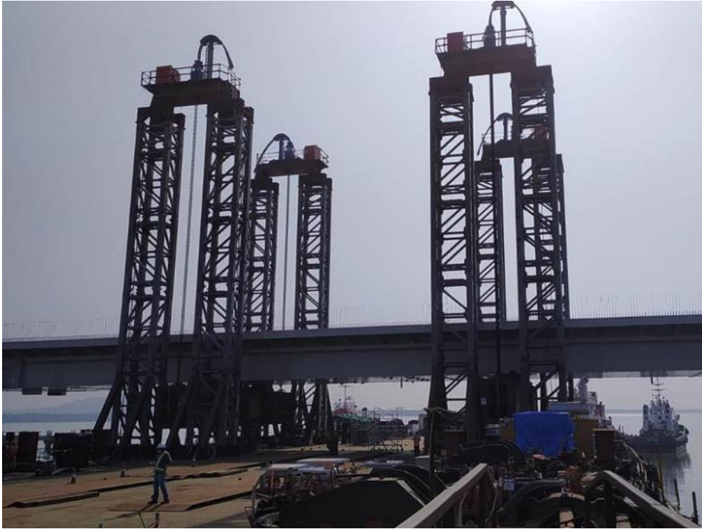
Photo No. 3: OSD lifted by Strand Jack for Load Test at Karanja Port in progress
