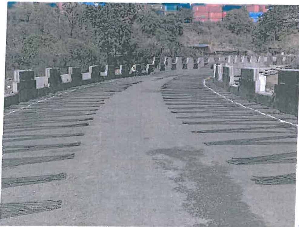
Photo No. 12: Chirle MJP Loop 2nd layer Geogrid work at CH 0+370 – CH 0+400
