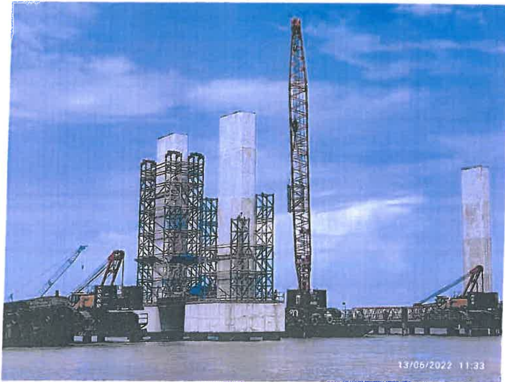
Photo No. 3: Integral pier head segment scaffolding at MP 188 RHS and LHS in progress
