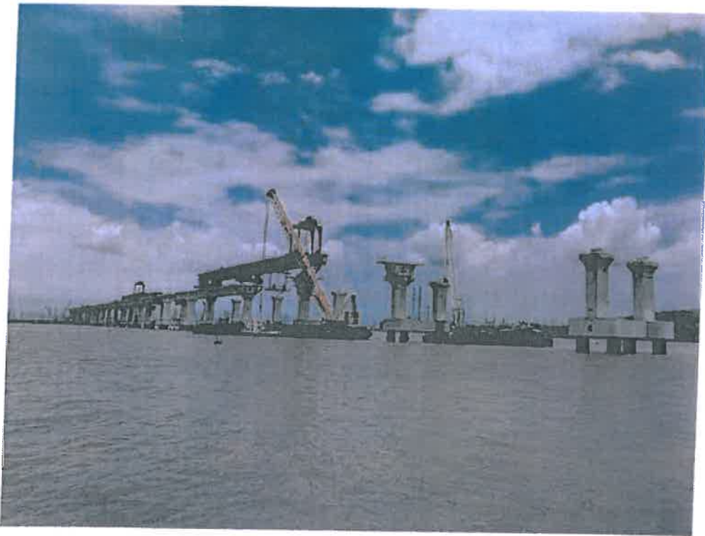
Photo No. 1: LG- 3 Span Erection at Marine Location looking towards Navi Mumbai
