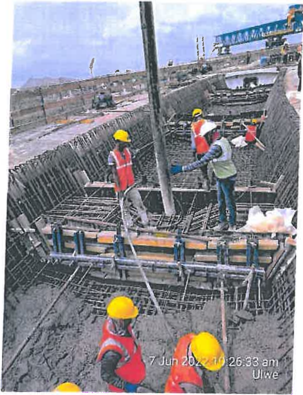
Photo No. 7: Cast in situ slab concreting at Interchange Area in progress
