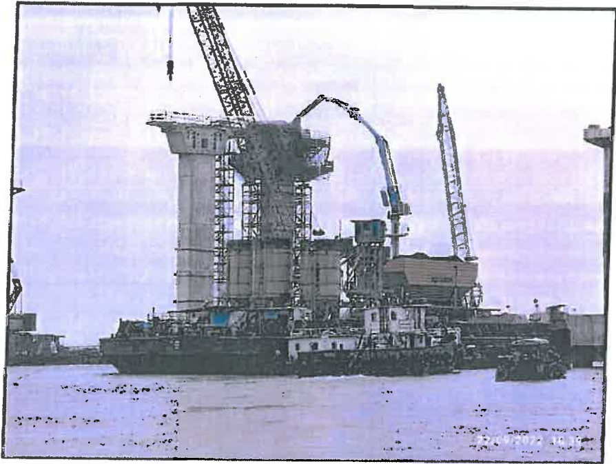
Photo No. 9: Integral pier head segment concrete at MP 190 LHS in progress
