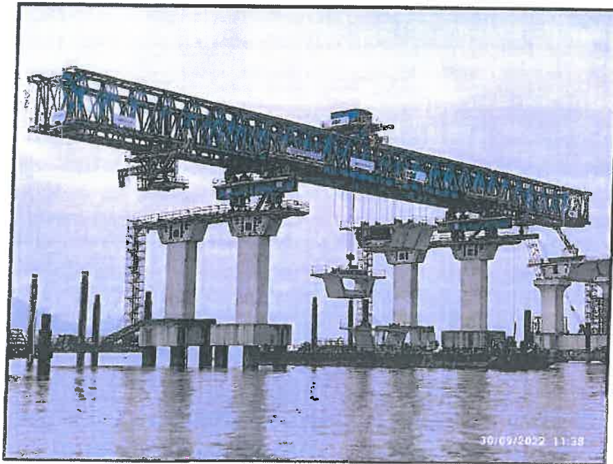
Photo No. 1: LG-1 Load Testing at MP 148A- MP 148B LHS in progress
