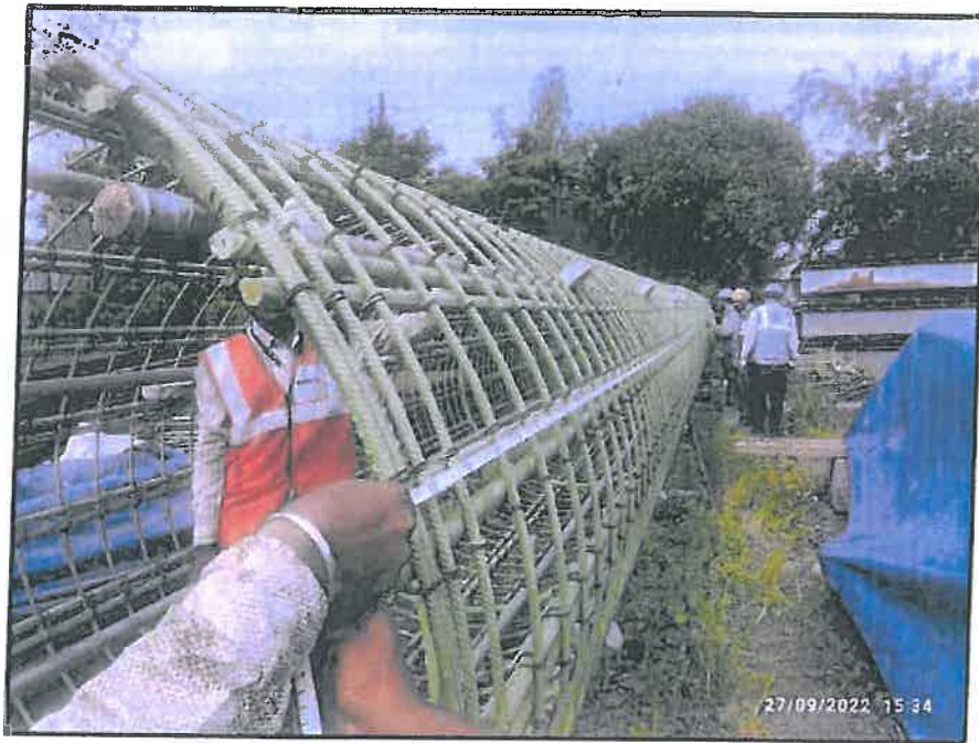
Photo No. 5: Pile reinforcement cage inspection at MP 240 R Substation in progress
