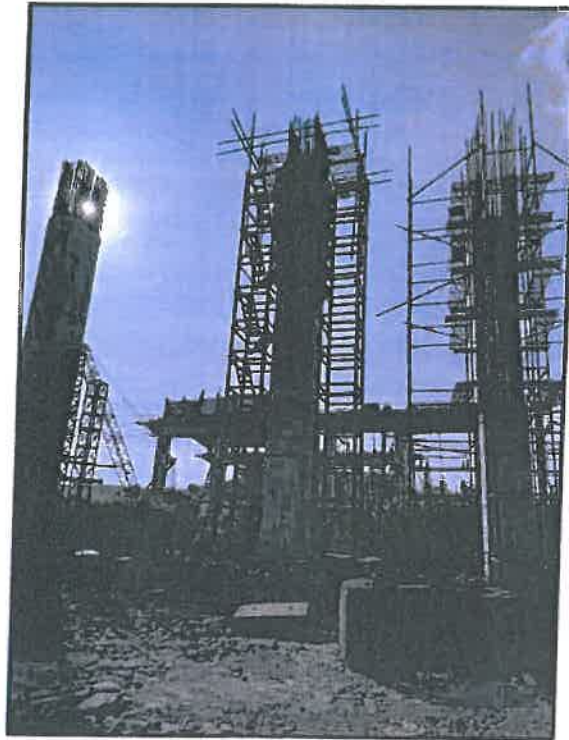
Photo No. 7: Chirle Pier RP 28 L final lift shuttering works in progress
