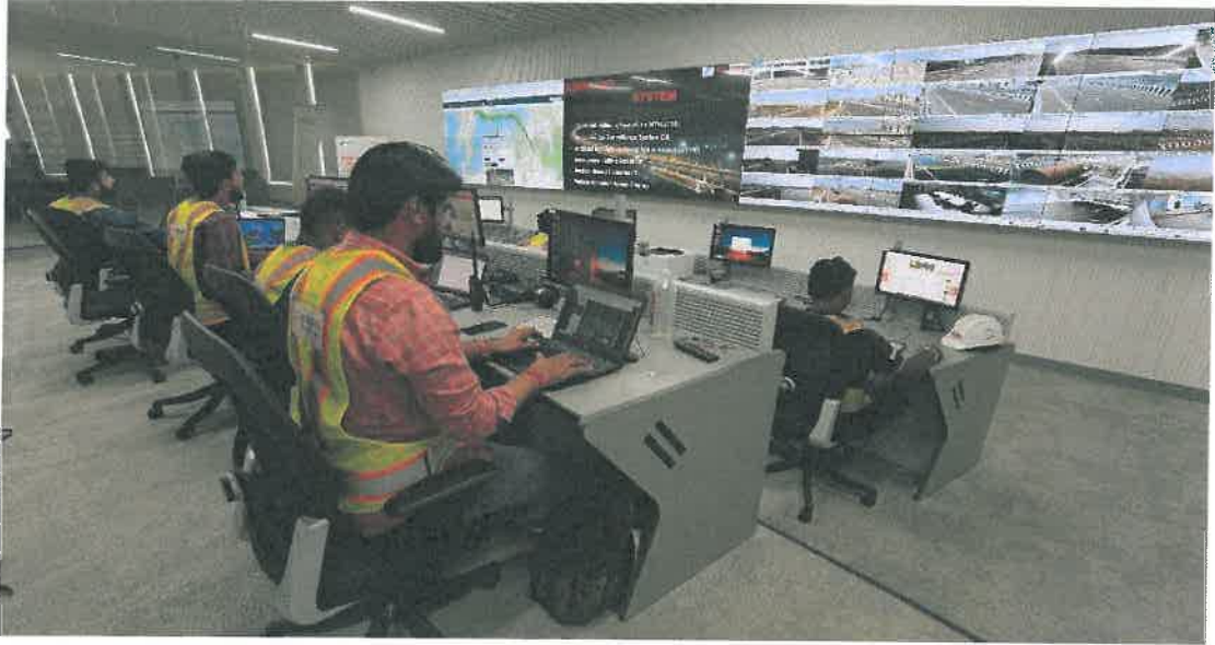
Photo 5,6,7- Photographs of Command Control Center
