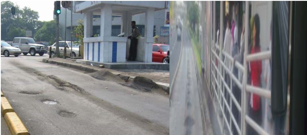
Figure 4. 9: Busway deterioration in Jakarta Figure 4.10: Concrete sections installed at stops
