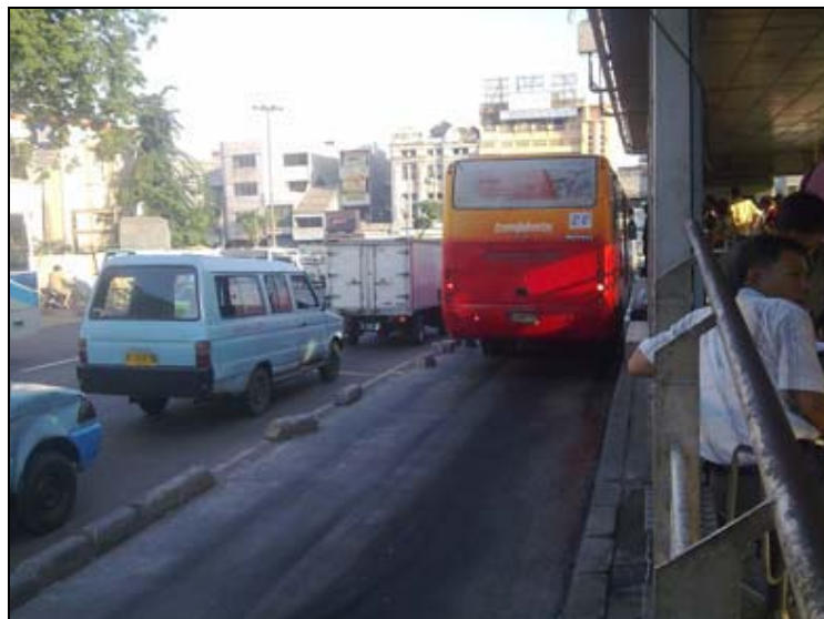
Figure 4. 11: Lane divider damage
